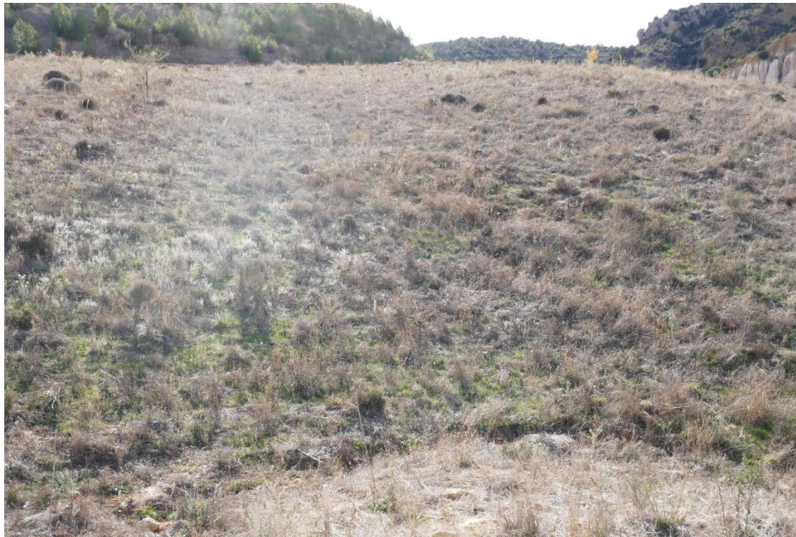
Figure 3. Detail of Western GeoFluv “Conventional GeoFluv with tree holes”. This is the main constructed slope with concave and convex forms. Rills formed in 2019 (photograph above) are not visible in the photograph below (December 2023), covered by vegetation and no longer functional.
