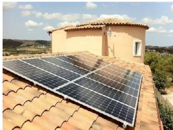
Figure 16. Photovoltaic Solar Installation in an Isolated Dwelling.
